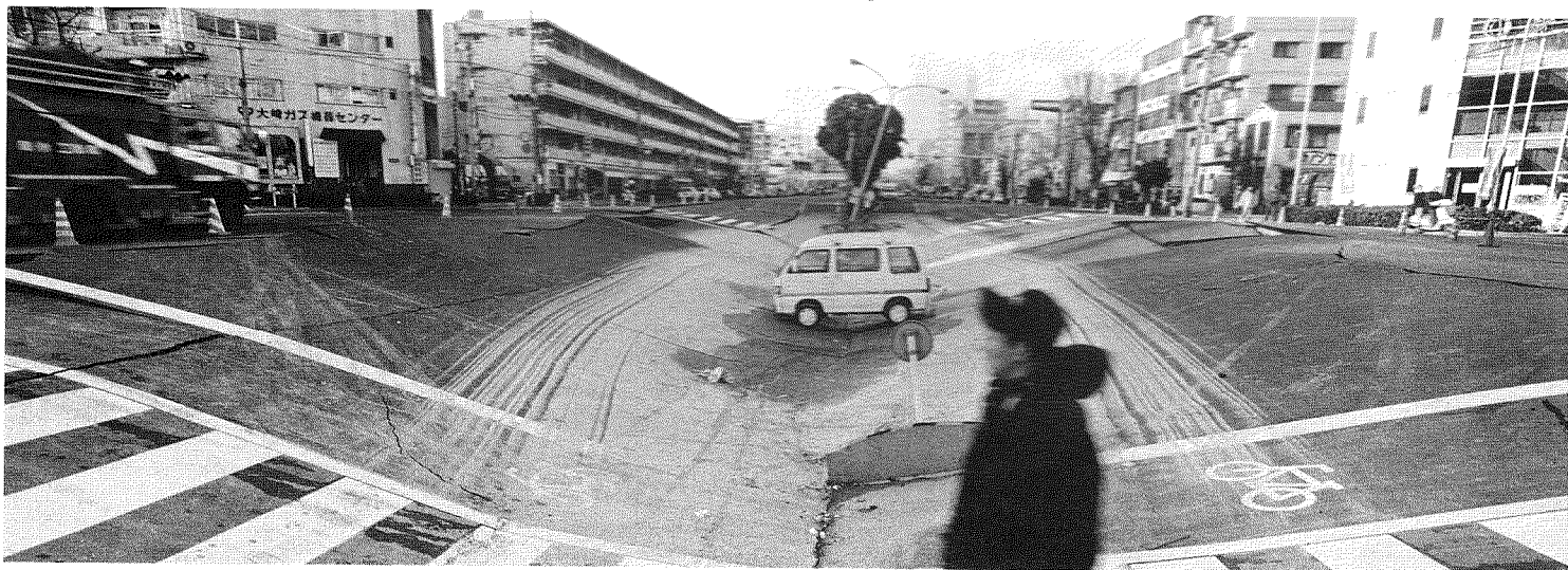
A man walks across a section of a road that collapsed above a subway station KIMIO IDA
